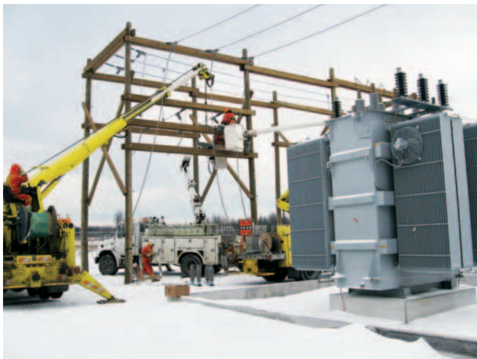
In 2007, a new $1.4 million substation was commissioned in Gananoque, providing improved reliability and security of service to the community.
