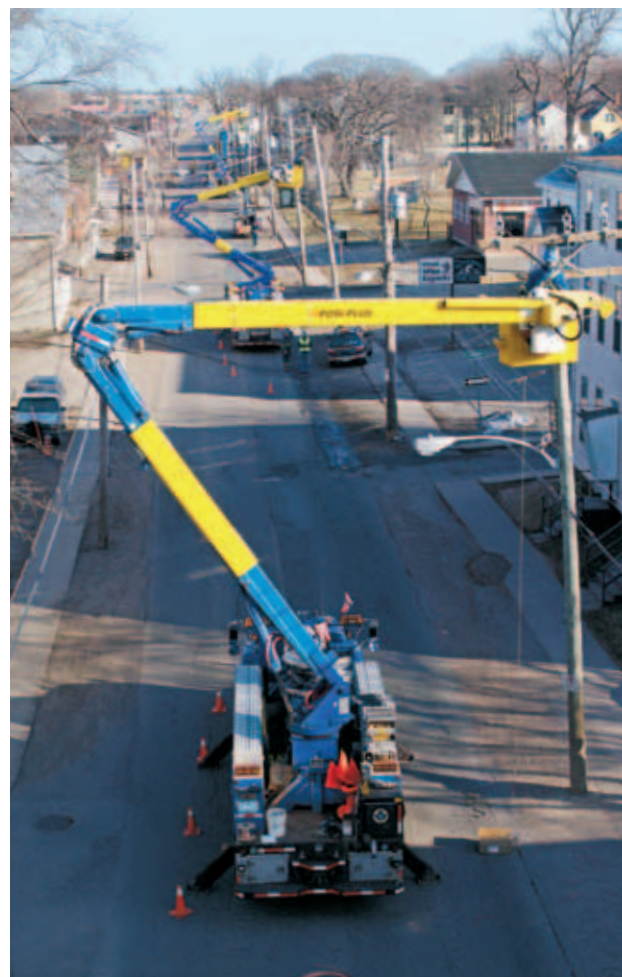
Maritime Electric invested approximately $27 million, before customer contributions, in 2007 to improve system reliability and customer service.
