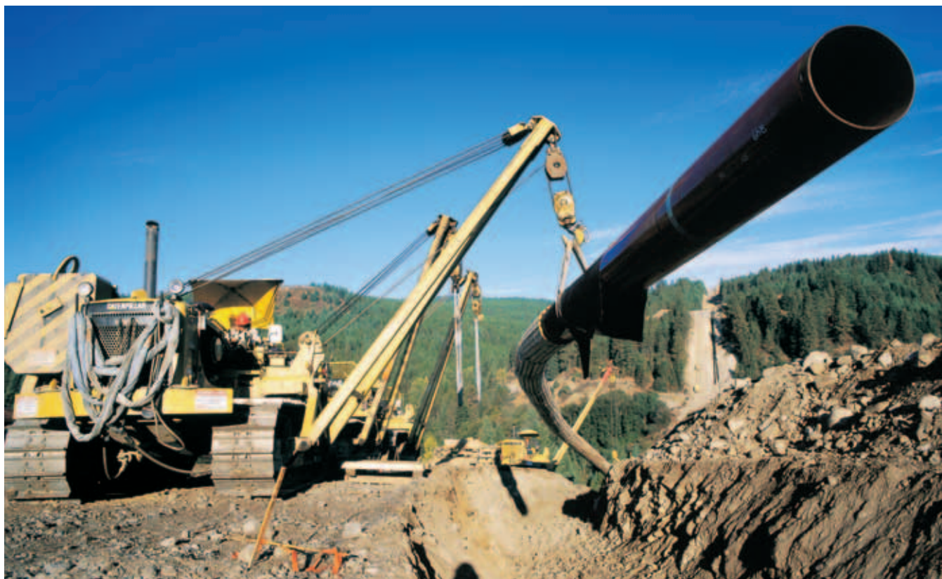
The Terasen Gas companies own and operate more than 45,000 kilometres of natural gas distribution and transmission pipelines.
