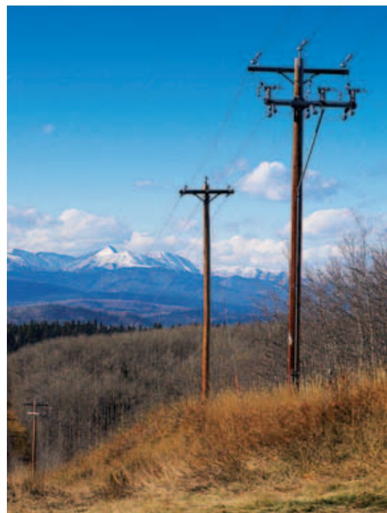
Fortis electric utilities own and/or operate approximately 134,000 kilometres of transmission and distribution lines.
