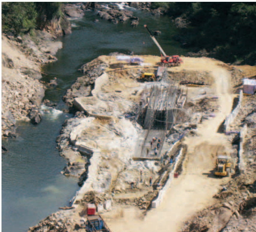
In May 2007, construction began on the US$53 million 18-MW Vaca hydroelectric generating facility situated approximately five kilometres downstream of Mollejon on the Macal River in Belize.
