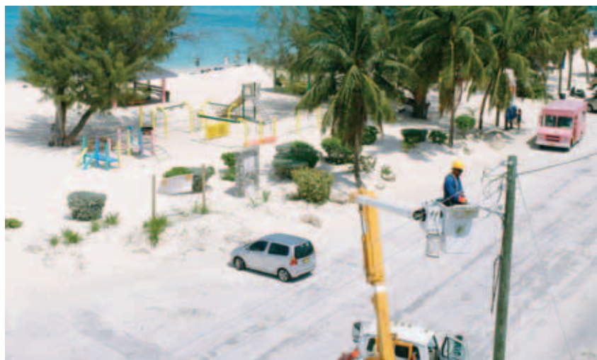
Caribbean Utilities owns and operates approximately 550 kilometres of transmission and distribution lines and 22 kilometres of high-voltage submarine cable.
